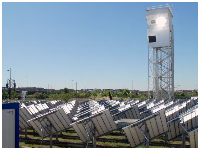
SUN-to-LIQUID research facility, Photo Credit: Christophe Ramage, © ARTTIC 2019
